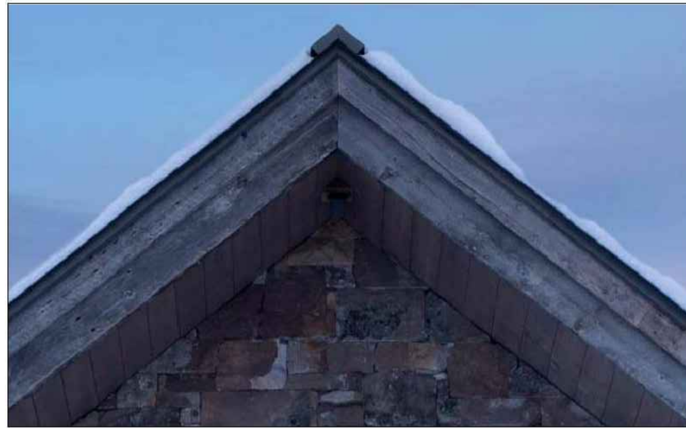
④ WEATHERED FASCIA AND STONE
